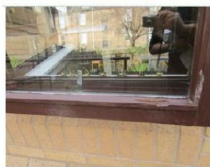
Timber repairs required to glazing bead
