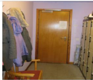
Staff changing room New flooring advised
