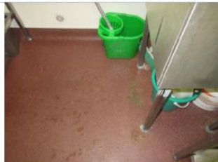
Commercial kitchen Some areas are stained and marked from footings of equipment, Deep clean advised
