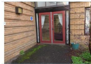
North Fire Exit door Moss and weeds should be removed from tarmac
